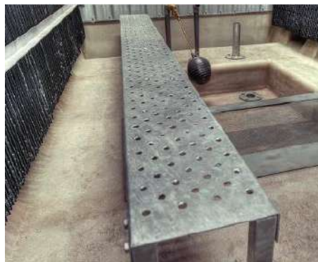
Internal Maintenance Walkway: (Optional Items)
